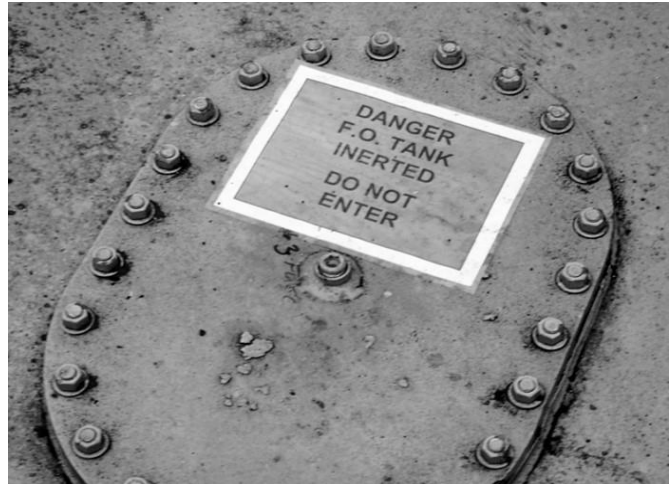
Inerted Tanks Must Be Posted Even Though Bolted Shut
