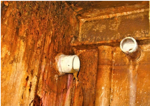
Biohazards in a Sewage Tank
